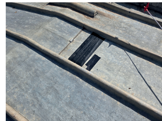
There are numerous patches
